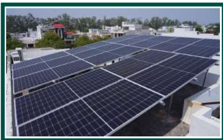
Residential Rooftop Solutions
